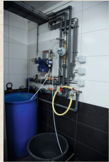
Water sanitation station
