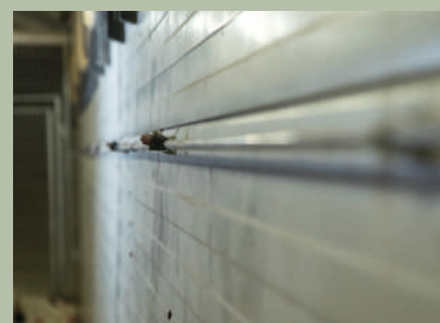
Fog installation in rearing house
