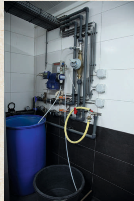
Water sanitation station
