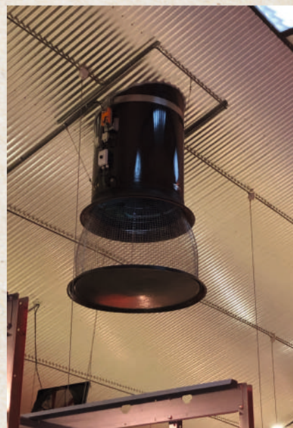
Under pressure climate control system in free-range barn
