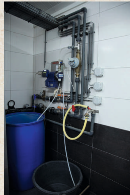
Water sanitation station
