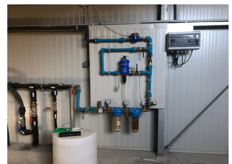
Water chlorination station
