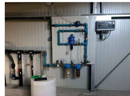
Water chlorination station
