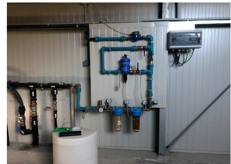
Water chlorination station
