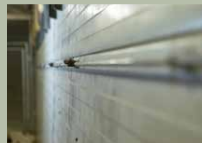
Fog installation in rearing house
