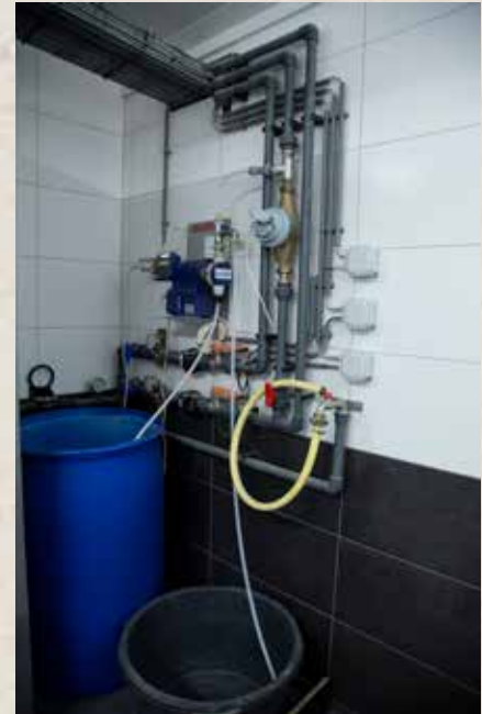
Water sanitation station
