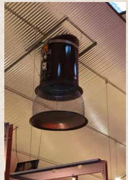
Under pressure climate control system in free-range barn
