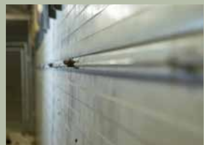
Fog installation in rearing house
